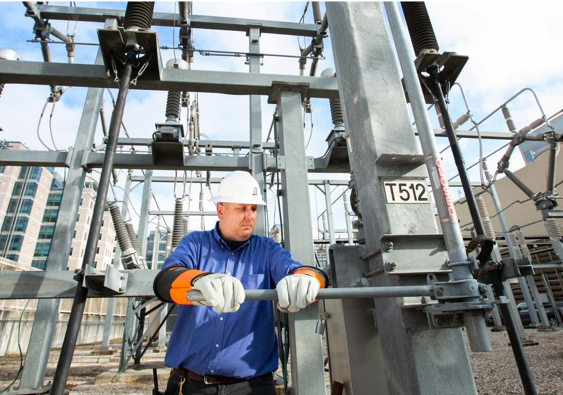
Brandon Johnson, shift supervisor, at one of TECO's two 138 kV local electric utility substations that feed grid electricity to TECO and also relay excess TECO-produced electricity to the grid when available.
