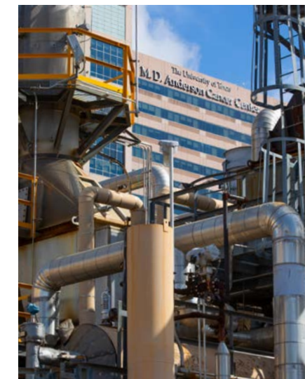
At left, Antonio Lopez, Jose Garcia and Jason Berrio with TECO's 48 MW combined heat and power unit.
